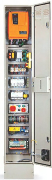
MRL Control Panel
